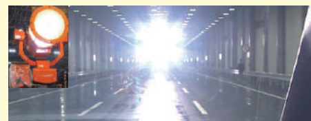
日照設備での点灯状況 Operational situation of sunlight device
