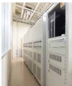
蓄電池充放電試験装置 Battery charging and discharging test apparatus
