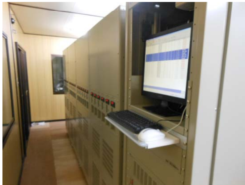
Charge/discharge testing system
